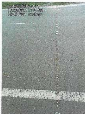
AE marks the defect
