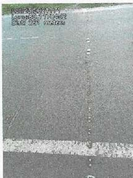
AE marks the defect
