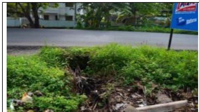
Choked culvert at 481.810
