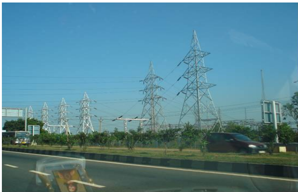
Electricity Power Distribution station along the existing Highway (NH-4)
