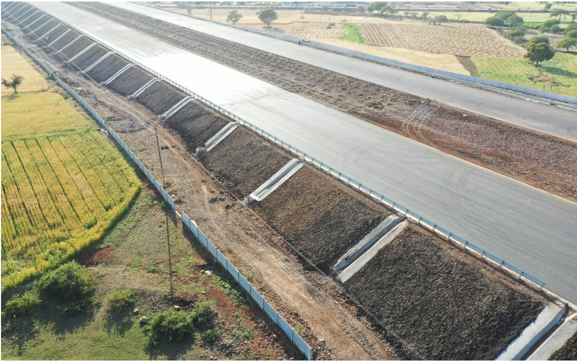
SMA completed near Ratlam, Madhya Pradesh
